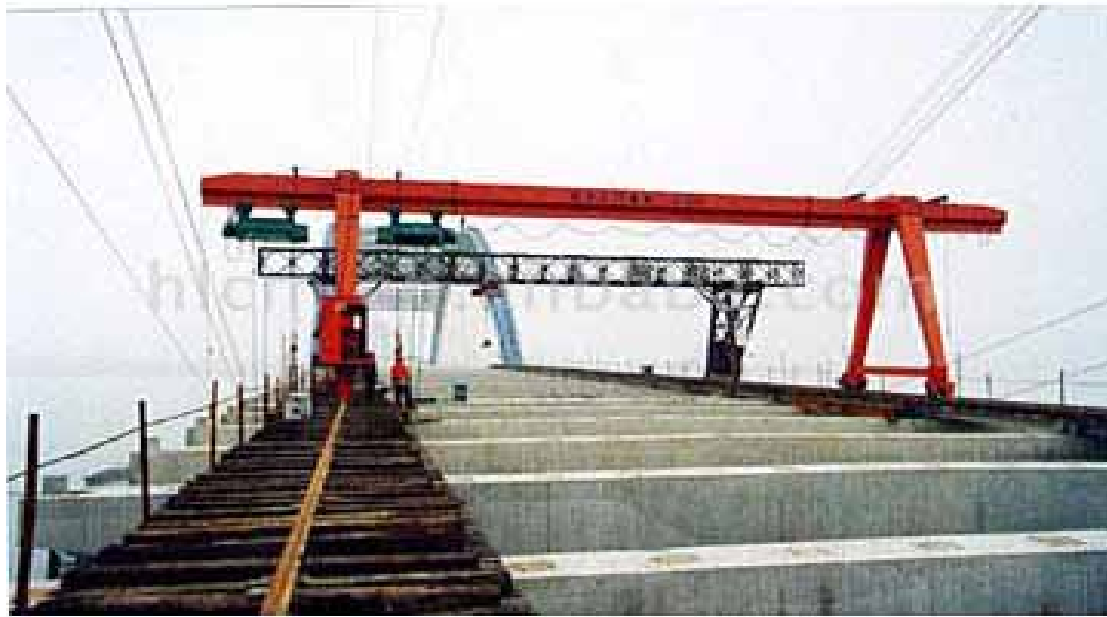
A gantry crane of the type that would be used for light maintenance
